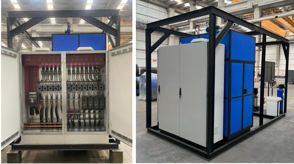
Figure Ap. 4.15 Electrical Control Board
